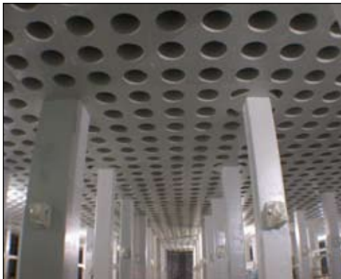
Series 215 Surfacing Epoxy was used to fill and surface over 500,000 square feet of concrete waffle slab at the new Samsung facility in Austin, TX.
