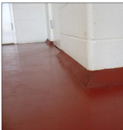
StrataShield's Ultra-Tread floor toppings were used to protect the concrete floors at the Hill Country Bakery in San Antonio.
